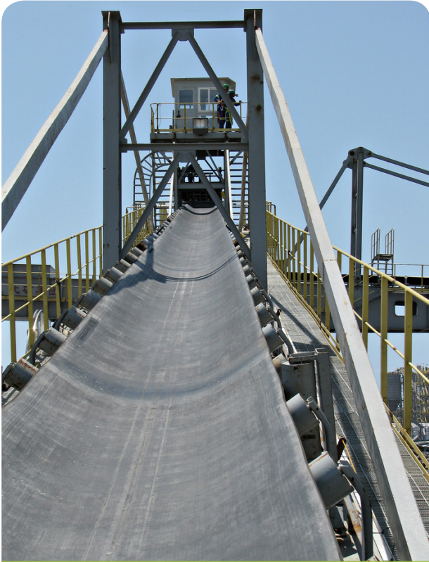
Rubber conveyor belt for loading
